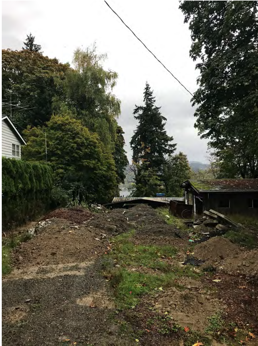
Exhibit 3-D: Second Stop Work Order Posted Photo taken 10/19/2020.
